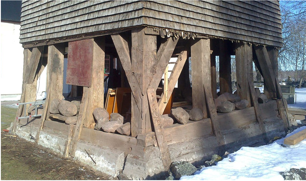
Fig 7. Ransbergs tower campanile. The secondary clamped sill with inner and outer plates.
